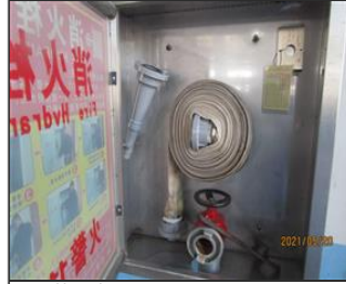
Photo of fire safety equipment Fire hydrant.JPG
