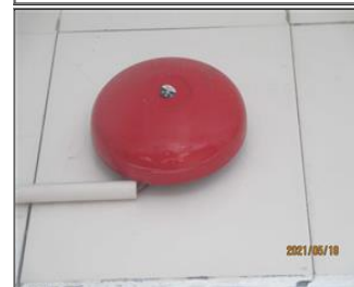
Photo of fire safety equipment Fire alarm.JPG
