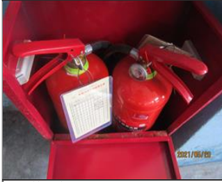
Photo of fire safety equipment Fire extinguishers.JPG
