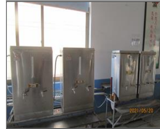
Photo of the sanitary facilities Drinking water.JPG
